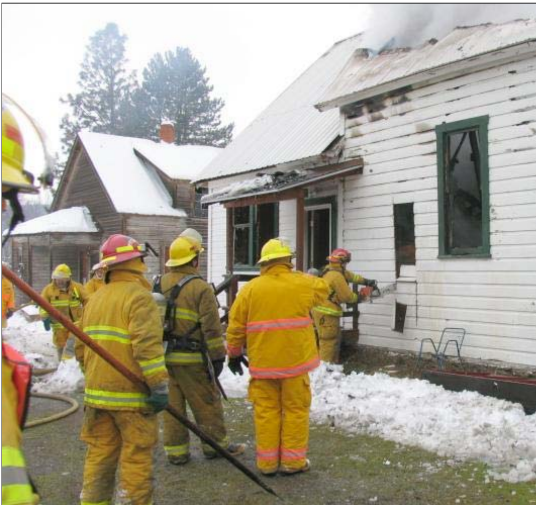
A chain saw is used to cut holes in some parts of the walls so fire fighters could get water on the flames.
