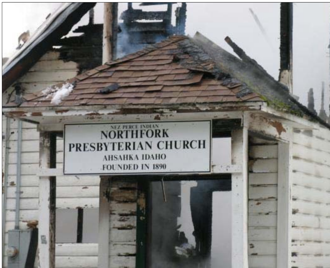
Nez Perce Indian Northfork Presbyterian Church was founded in 1890. The structure stood near Dworshak National Fish Hatchery, east of the North Fork of the Clearwater River.
