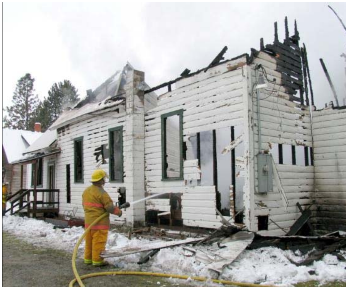
A fire fighter sprays water on flames through a hole cut earlier with a chain saw.
